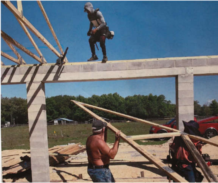
Mayor Goodman helps lift a roof truss at the Williston Animal Shelter construction site
