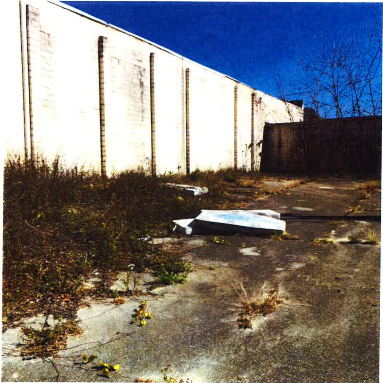
1050 NE 6th Blvd, Richardson Property Remains in Non Compliance.
